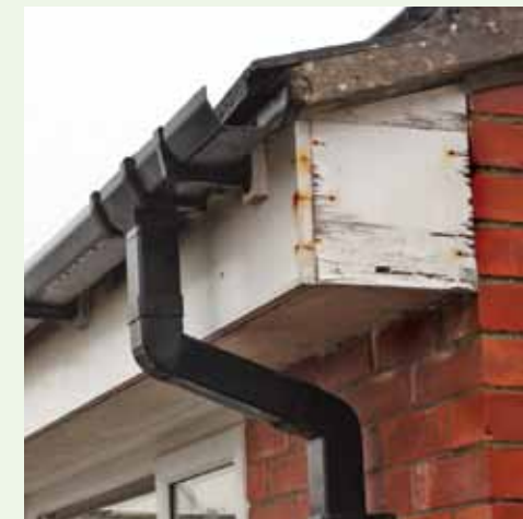
Timber roofline can rot without maintenance...
